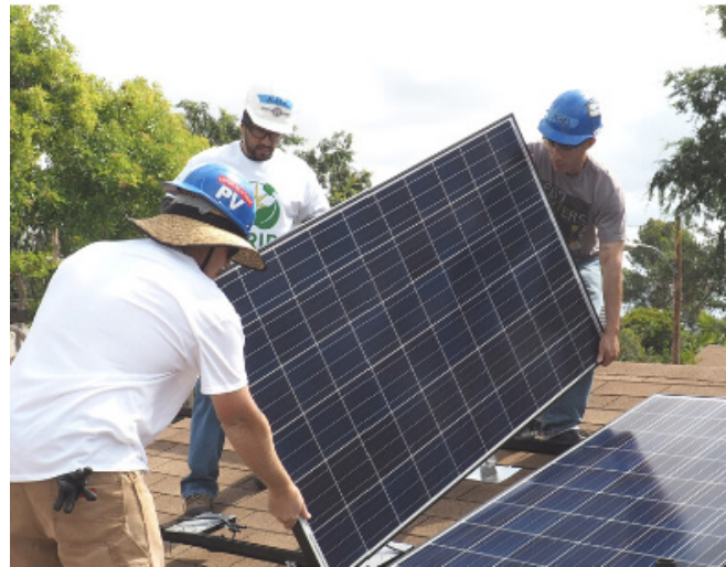
Solar installation for LIWP project (Credit: CSD)
